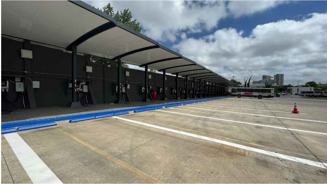
Photograph 5 Existing chargers Añón Plant
